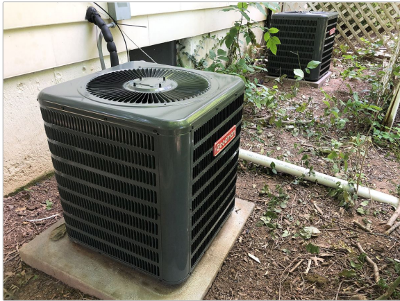
Condensing unit, north side
