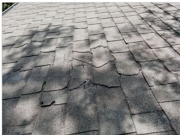
Granule loss and curling, south slope
