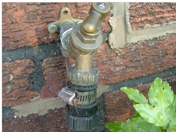
South wall hose bibb
