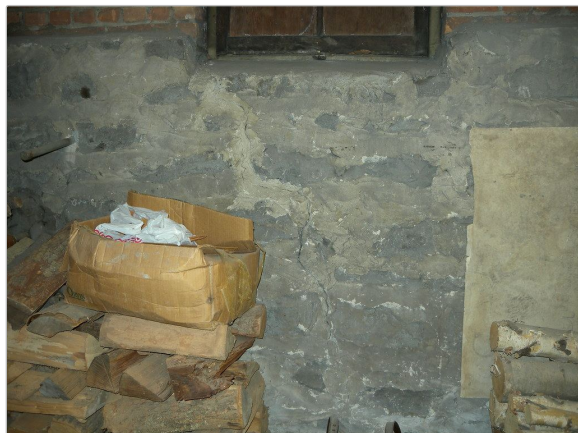
Vertical crack, northeast wall
