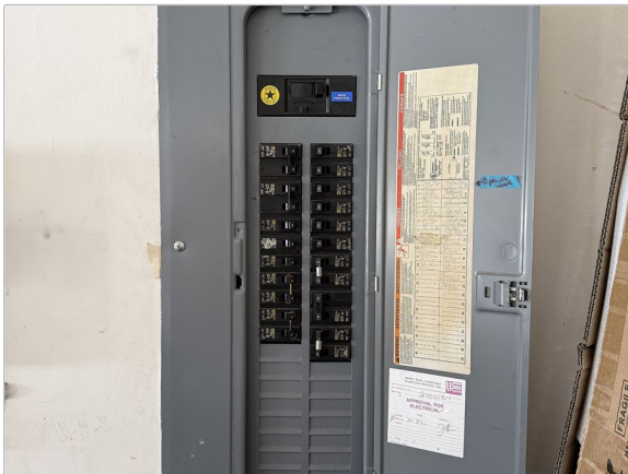
200-amp main panel, basement
