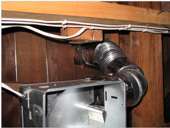
Hall bath exhaust fan duct in attic
