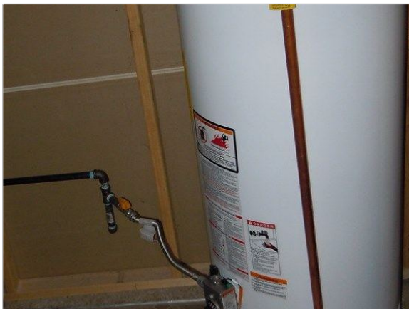
50-gallon gas water heater
