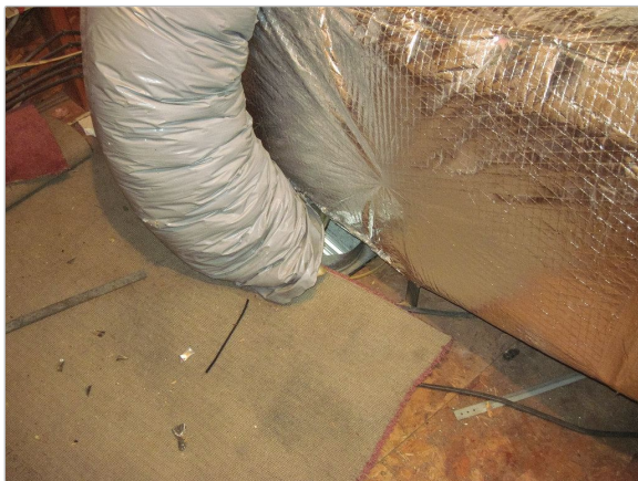
Kinked flex duct at register boot
