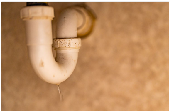
Drip at trap slip joint, hall bathroom
