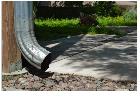
Downspout discharging at rear foundation
