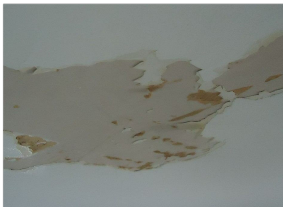
Stain at dining-room ceiling below hall bath
