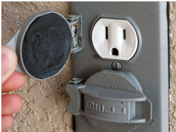
Rear patio receptacle
