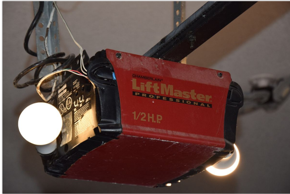
Overhead door and opener
