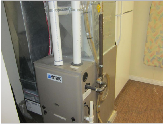
Forced-air gas furnace
